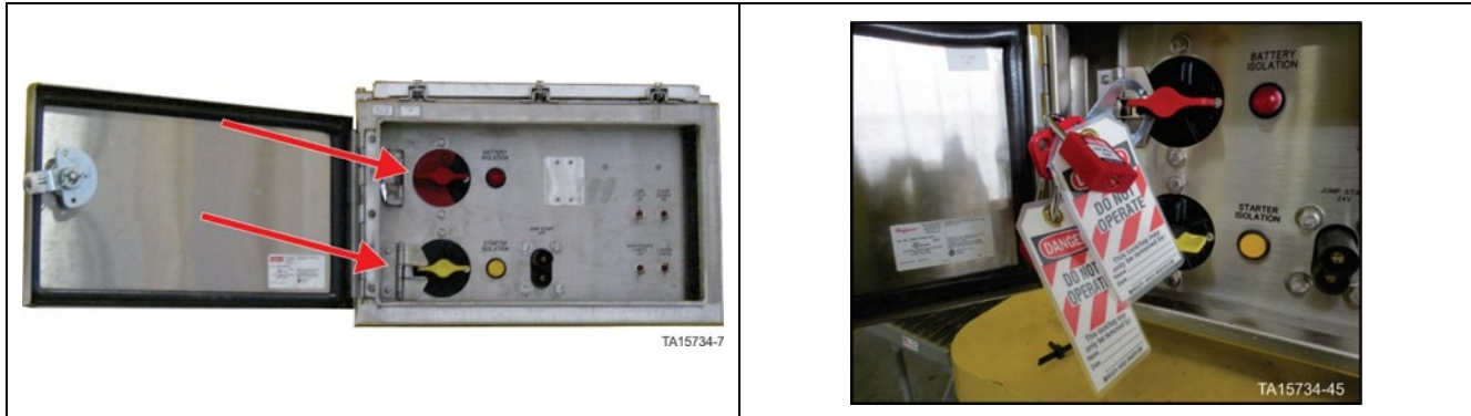
Figure 3. Battery Isolation Box – Battery isolation switch in OFF position with locks in place
