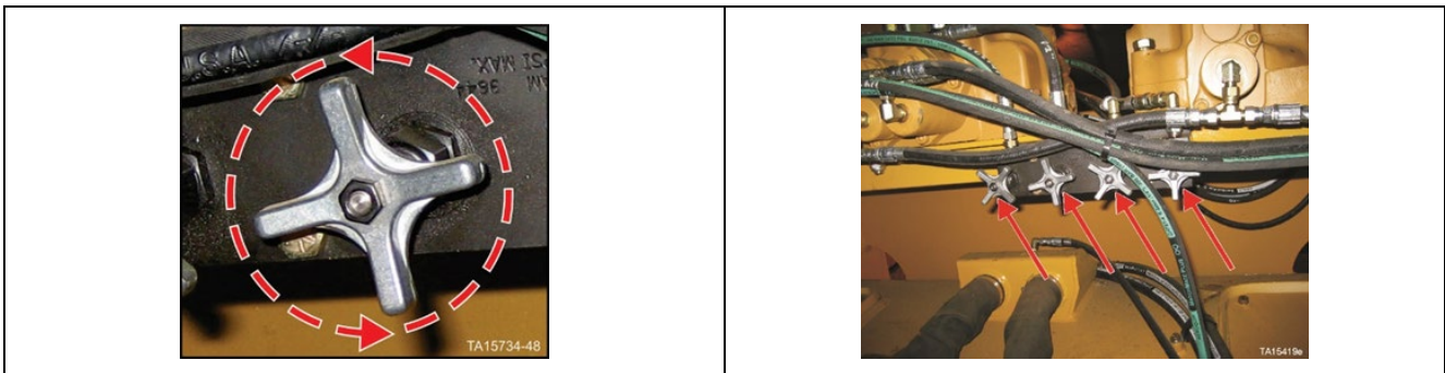
Figure 6. Pressure bleed down valves
